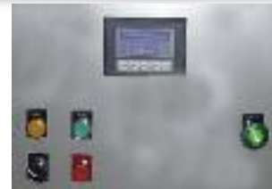
Control panel detail
