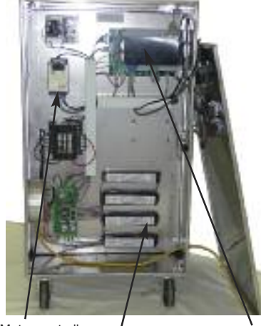
Motor controller Ballasts PLC computer
